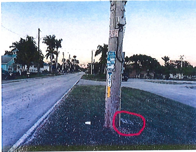
Pull box to be adjusted, 67+20 Rt
